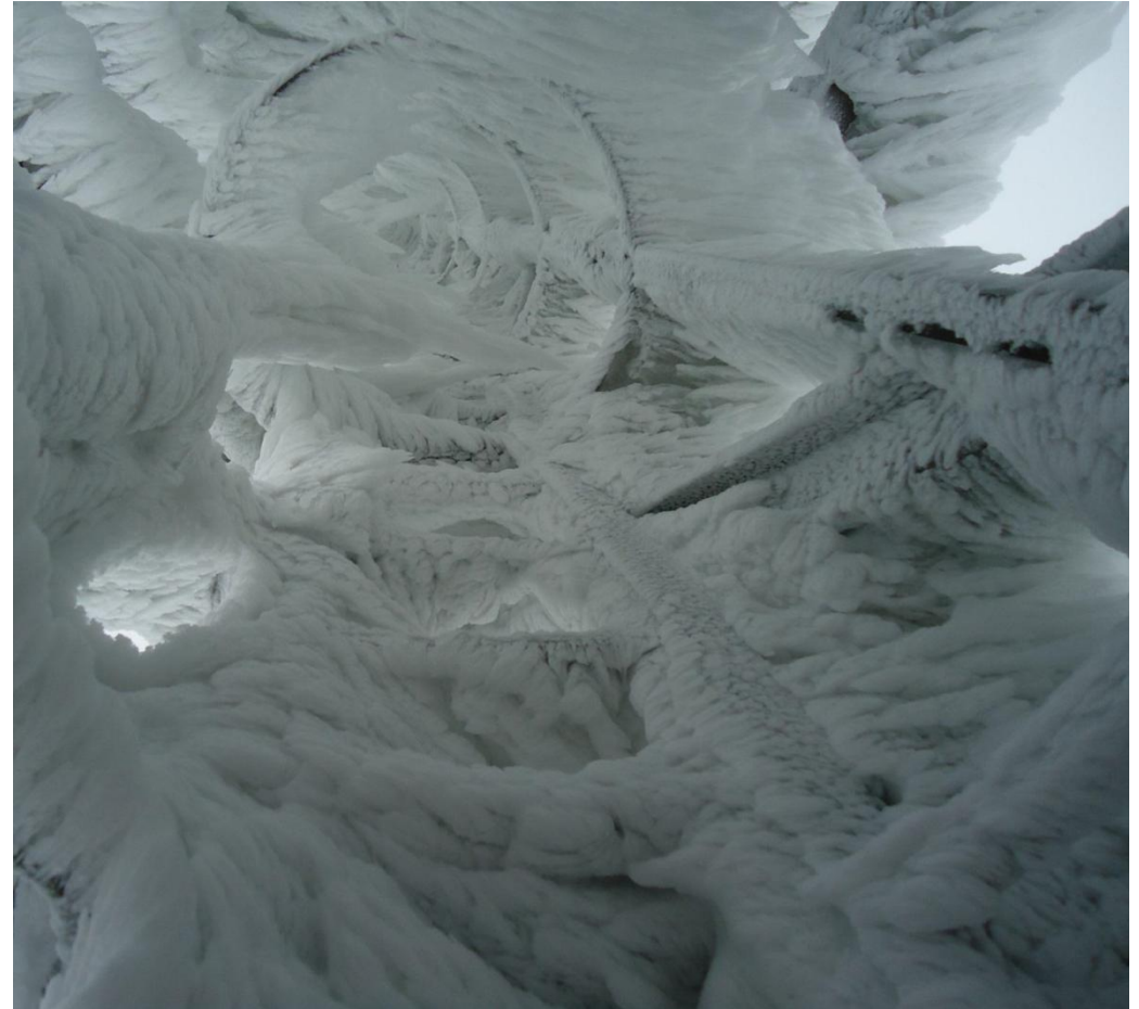
Example of accumulated ice at Tryvann communication mast, Oslo, 2014.
